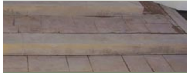
Before old, discolored concrete
